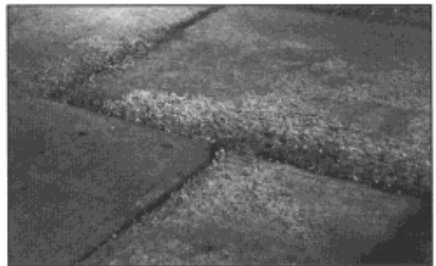
Scaling concrete surface
